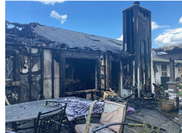
(Maureen Ct. Structure Fire)
